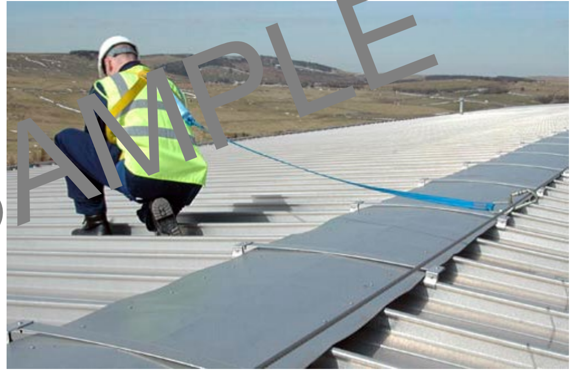
Use of a work restraint system to prevent worker going near unprotected edge
