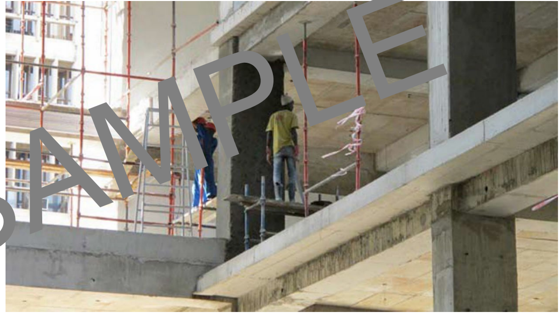
Working at unprotected edge
